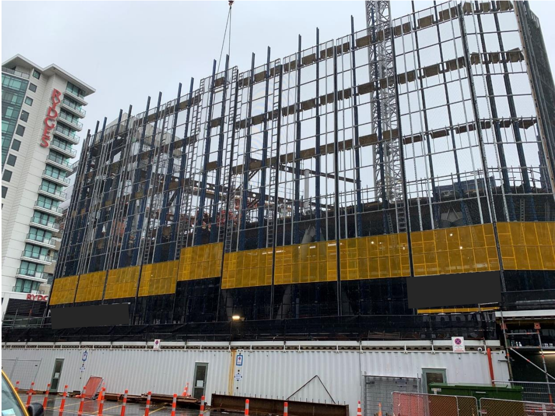
Figure 1-53a: Photo example of screens
