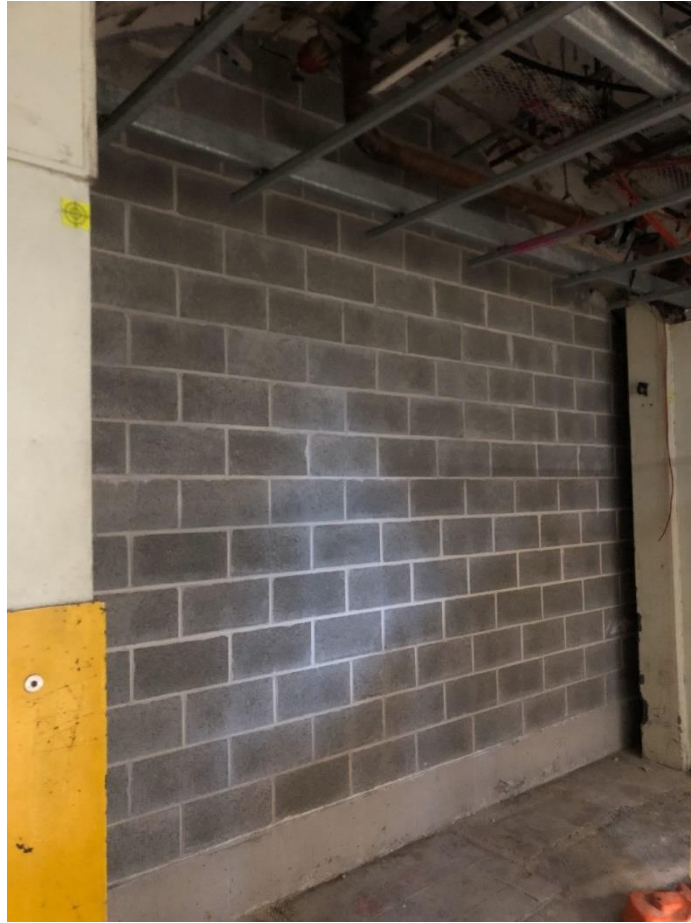
Figure 1-21: A-Class Hoarding – South-Western Baggage Tunnel
